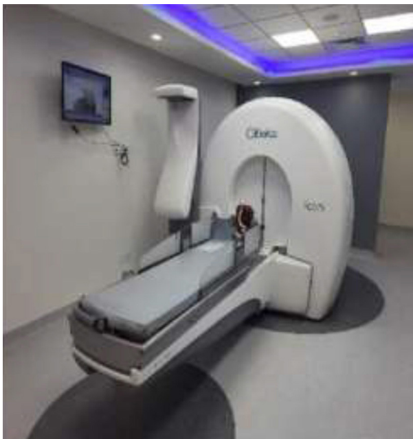
Fig. 1. Elekta Icon Gamma Knife machine installed at our center
